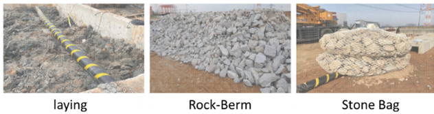
Fig. 9. Safety facilities for HVDC cables.
